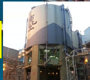
Raw PFA silos - Buffer storage for raw PFA
