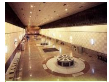
1200MW * 50%+ Guangzhou Pumped Storage Power Station
